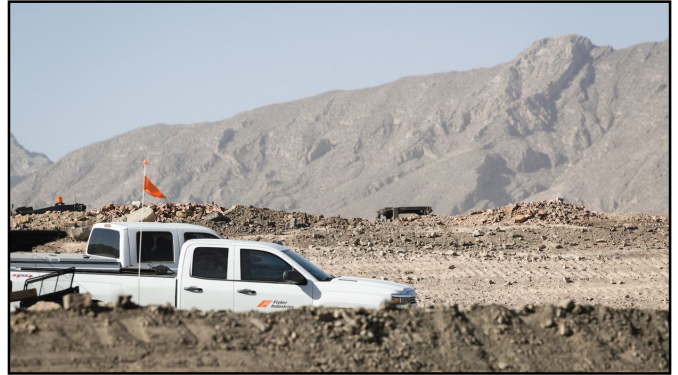
Trucks from Fisher Industries prepare the ground for a wall to be built on private property near El Paso, Texas.
